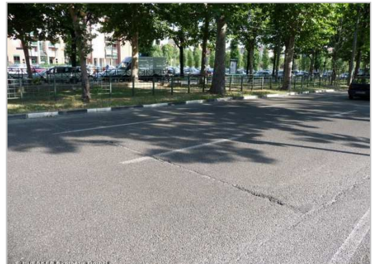
Fig. 7: Unreinforced area in July 2009
