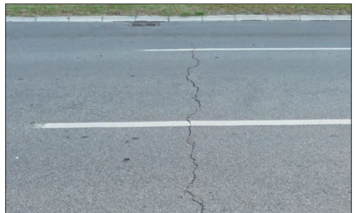
Reflective crack in an asphalt surface course
