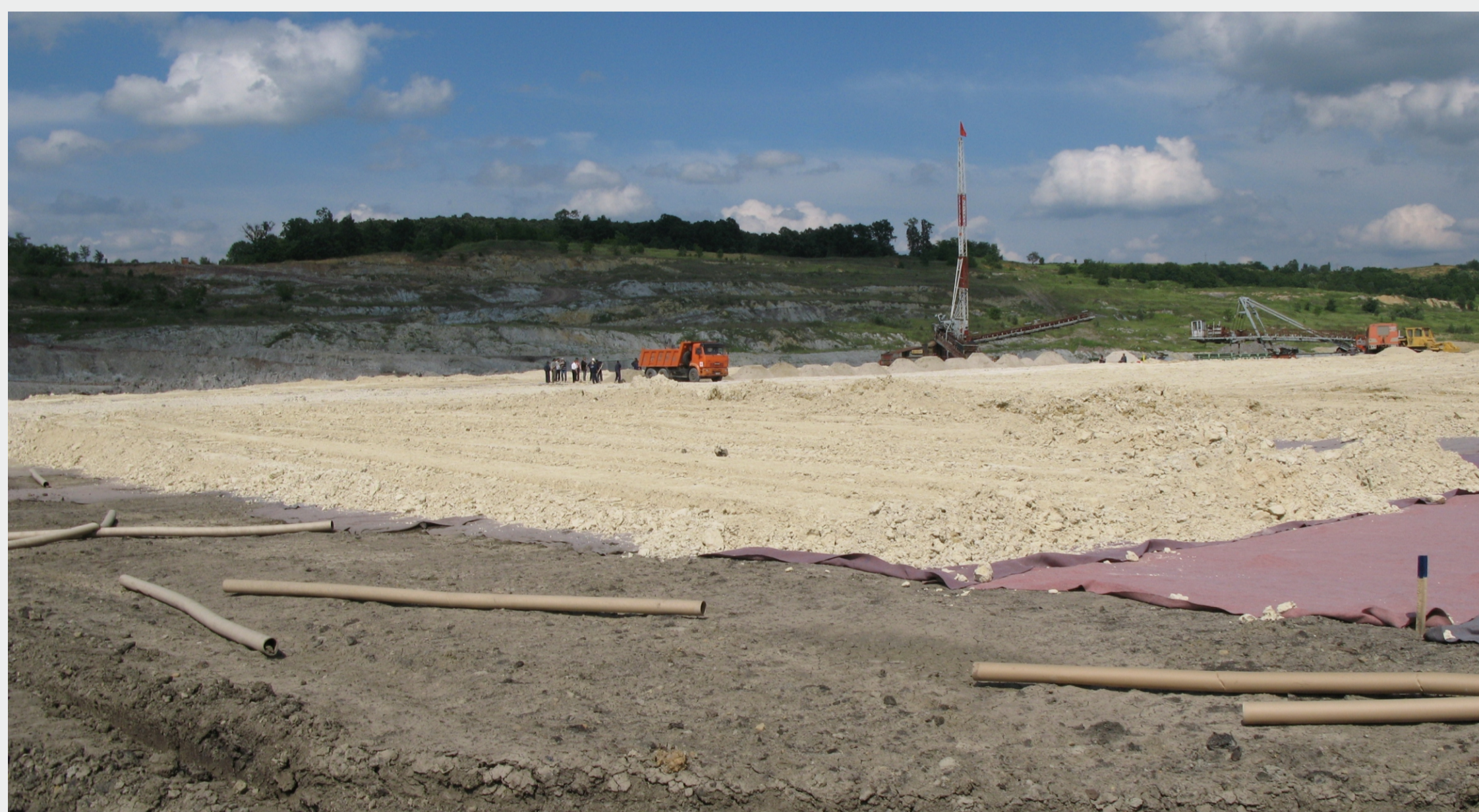
Base preparation: levelling of surface, installation of non-woven, placement of 20 cm sand layer
