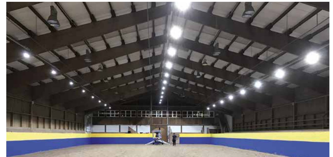
Optimal training and tournament conditions through the use of Lubratec LED luminaires.
