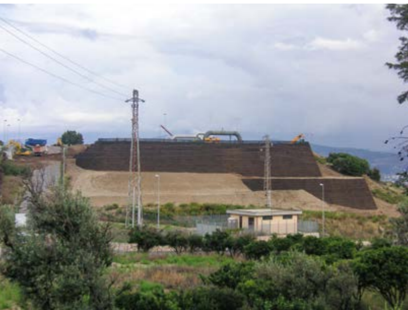
Modernisation of gas compressor station Italy: construction of extra-steep, low-settlement and settlement resistant slopes using geosynthetic reinforced soil method.
