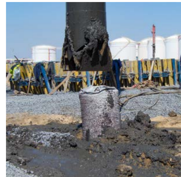
Ground improvement for oil tanks Spain: construction of safe, ductile foundation system in very soft soils with Ringtrac geotextile-encased columns.
