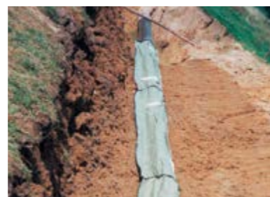
2006 Pipe cover, France, gas pipeline
