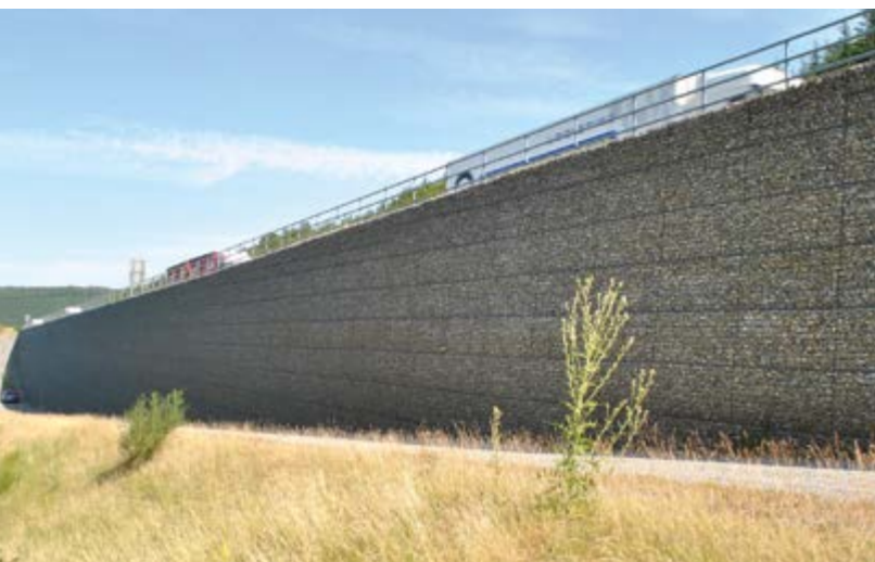
A3 motorway widening, Frankfurt/Main – Würzburg Germany | Embankment widening for new six-lane motorway sections east and west of Haseltalbrücke bridge – Up to 13 m tall full-gabion walls – Self-supporting GRS retaining wall with purely cosmetic gabion facing (passive construction).
