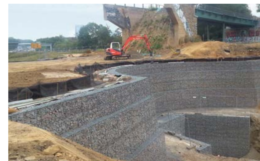
Uncovering of River Schondelle Germany | Sub-project of River Emscher ecological improvement scheme – Earthworks built with integrated lost formwork and full-gabion facing – Solution as replacement for originally planned concrete cantilever wall – Erected in three, 5 m tall vertical sections.
