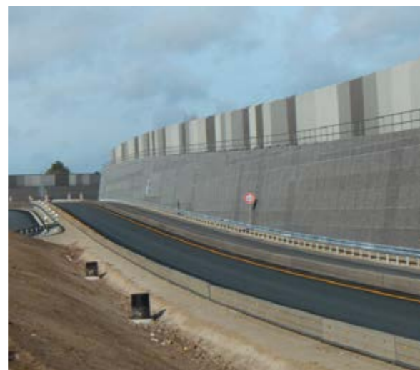
Highly absorbent noise barrier Germany | New highly absorbent noise barrier for six-lane widening of A3/A73 motorways, Fürth-Erlangen – Absorption category A 3 (sound absorption DL_a \geq 8 - 11 dB) – Gabions facing carriageway and vegetation on the other side – Height up to 10 m.
