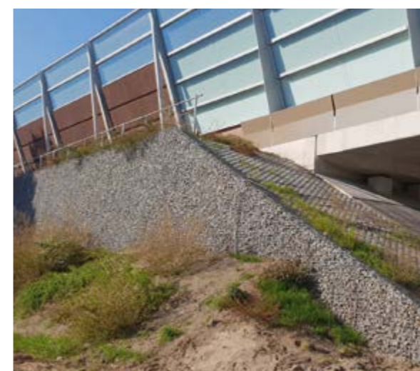
Motorway widening within existing footprint Netherlands | Six-lane widening of (A1/A27) motorway section near Utrecht – Natural sloping motorway embankment rebuilt as steep slope with Fortrac Gabion tie rod system – Erection of top noise barrier made possible by integration of concrete pile supports in system.
