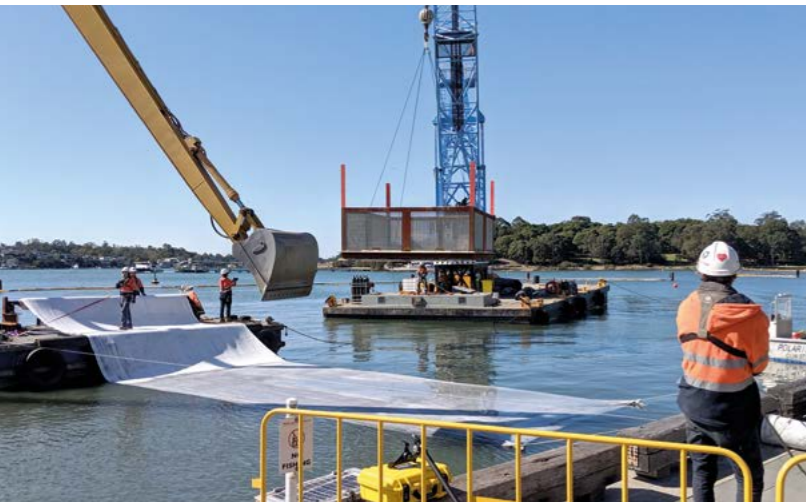
Securing of contaminated sediments Australia | Securing sediments with high PAH and CHC contamination in a Sydney bay. Installation of approx. 5,000 m 2 of Tektoseal Active AC as a pollutant barrier layer for improving the water quality.
