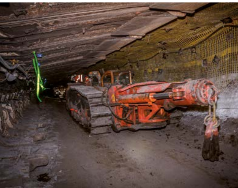
Powered Roof Supports (PRS) in Final position with Dozer preparing to safely remove PRS from face.
