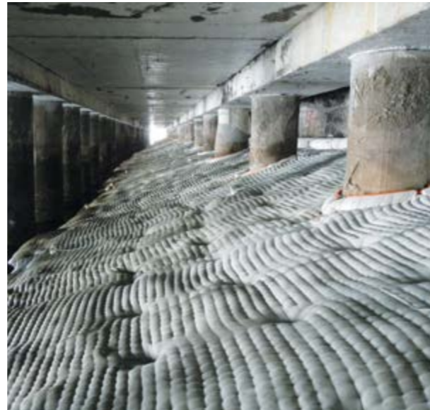
Bed protection Guatemala, 2016, slope and bed protection at new Quetzal port terminal using Incomat Standard.
