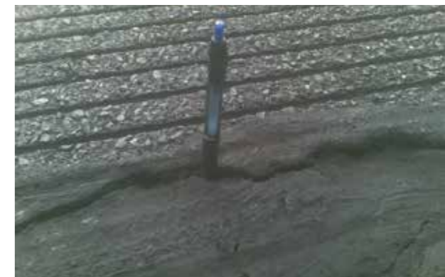
Pavement condition in 2009 prior to rehabilitation
